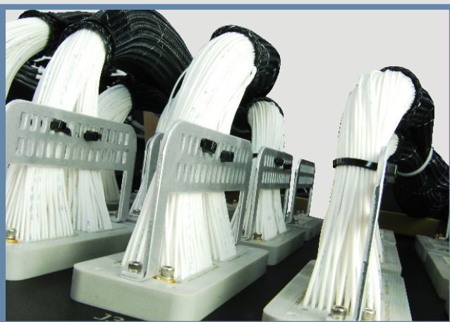
Cabled Connection with 24 awg cables
